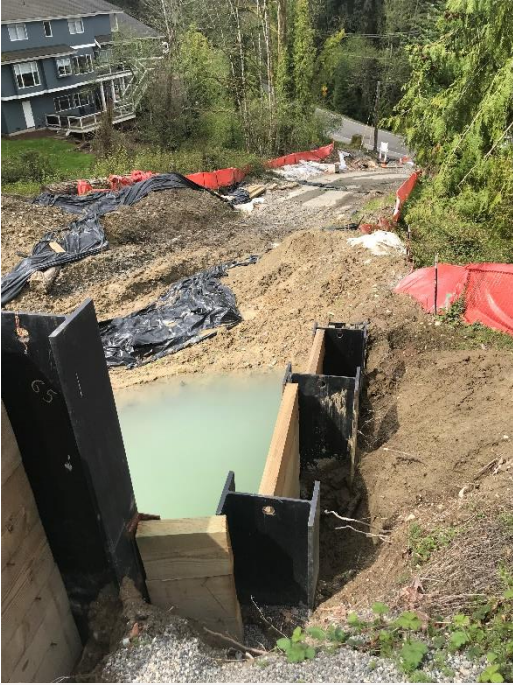
Photograph 4. Looking west from northeast corner of site down driveway to W Mercer Way. Temporary settlement pond below shoring wall
