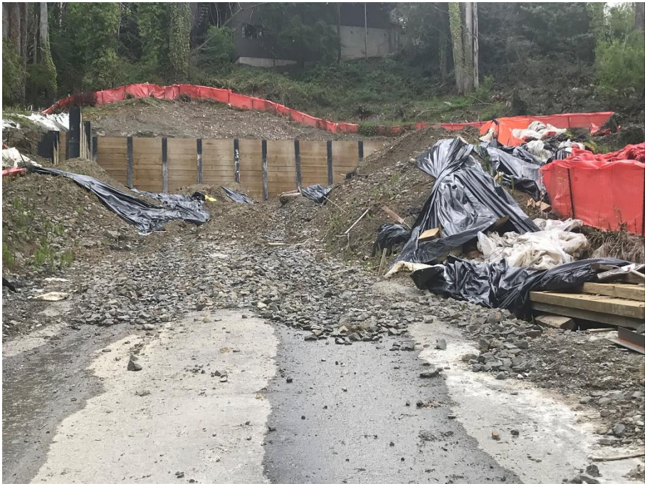
Photograph 1. Looking east up the driveway at shoring wall and cut slope above.
